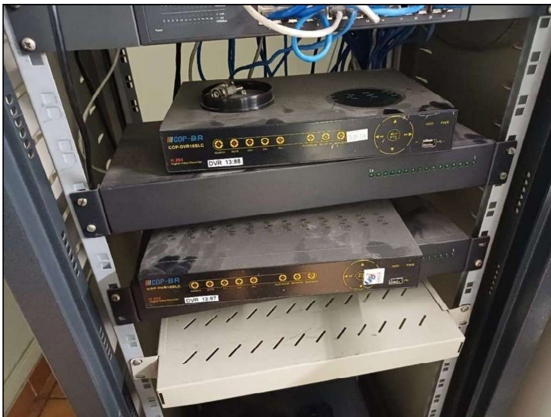
ITEM 015 - RACK COM 3 SWITCHES E 2 DVRS
