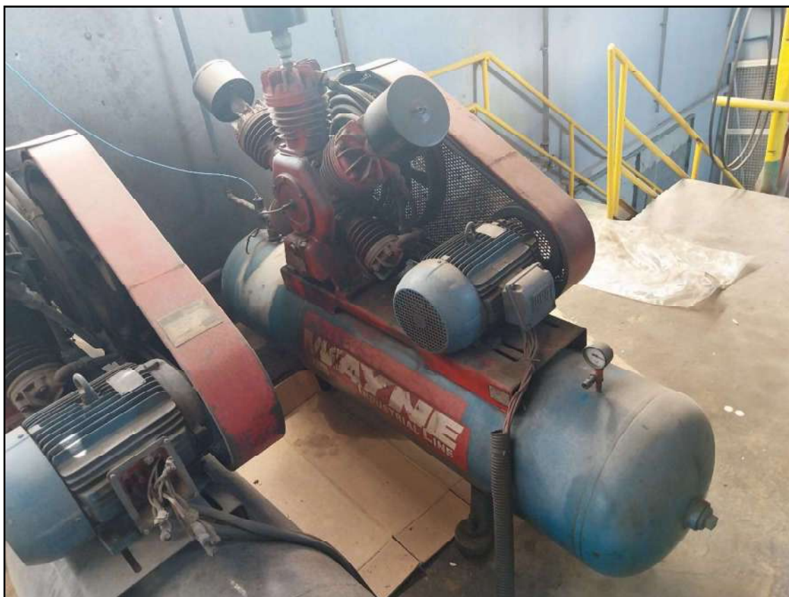
ITEM 083 - COMPRESSOR WAYNE LINE
