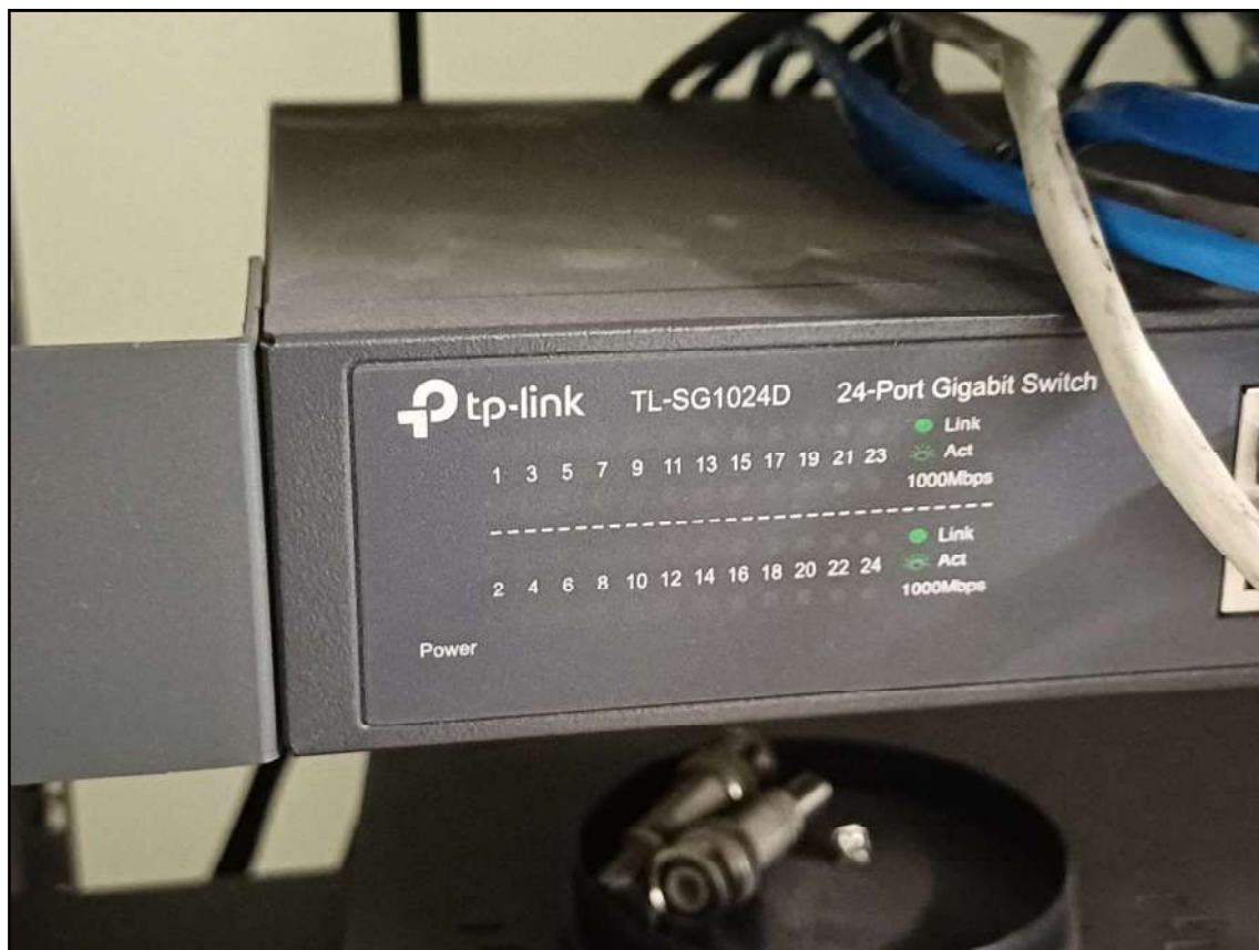
ITEM 015 - RACK COM 3 SWITCHES E 2 DVRS
