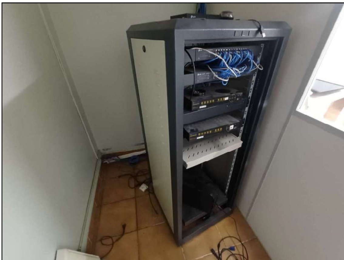
ITEM 015 - RACK COM 3 SWITCHES E 2 DVRS
